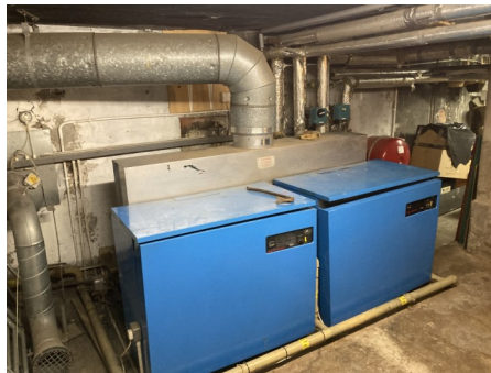
The old boilers have served us well
