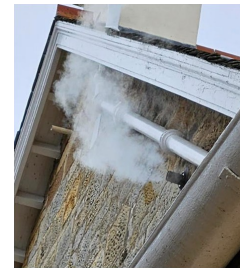
This boiler is wasting a lot of gas
